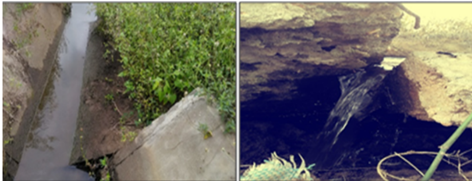
Figure 4 : Photographs illustrating the degraded main channel (breaks and cracks)
